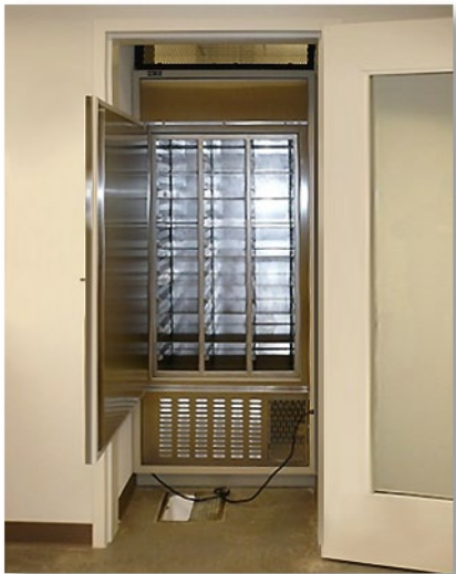
EXAMPLE 10C: Pass-through Temporary Refrigerator (Open rear view)
